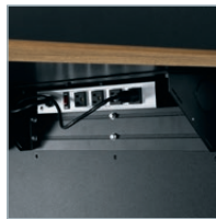
SECURE POWER DISTRIBUTION
